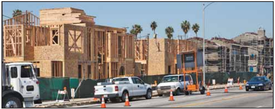
The Coronado in Long Beach, seen here under construction, is the latest new residential community that plans to revitalize the Atlantic Avenue corridor with affordable housing. The development includes for-sale townhomes and 2, 3 and 4 bedroom flats, featuring distinctive Spanish architecture. (Photograph by the Business Journal's Thomas McConville)
