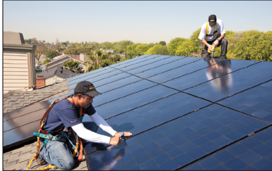
Solar Panels – Workers from AMECO Solar Company check the installation of solar panels on a home. Solar energy is expected to expand under current California laws mandating greater use of renewable energy. (Photograph by the Business Journal's Thomas McConville)
