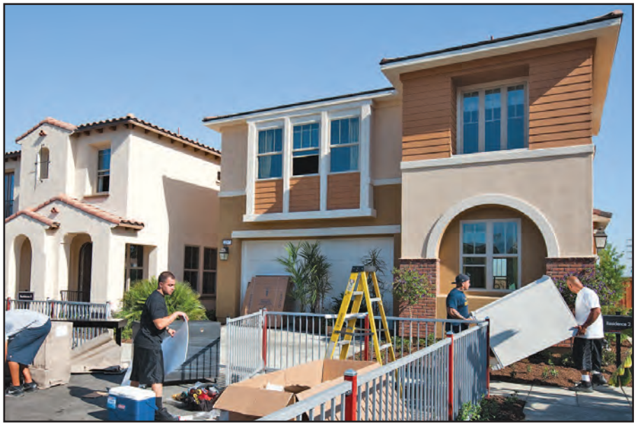
The Aubry at Alamitos Ridge residential development is quickly taking form at View Ridge Drive and Redondo Avenue. It’s the newest residential construction currently in Long Beach with 14 acres of 85 new homes or detached condos. Construction is expected to be completed by September. There are four designs of the two-story homes as part of Lennar Home’s PowerSmart Solar Home system design, which comes with solar panels, tankless water heaters and other energy efficient functions for residents to save money on energy costs. The above models are available for viewing. (Photograph by the Business Journal’s Thomas McConville)
